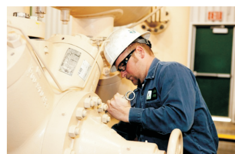
Travis Shull of Lodi Gas Storage L.L.C adds another day of injury-free work to their safety record (Photo courtesy of Mary Gillespie-Frazer)
